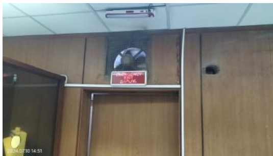
Exit sign & light.jpeg
