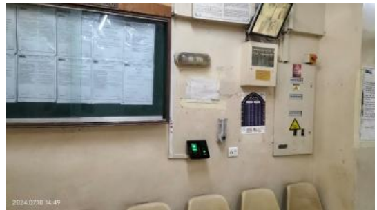
Fire alarm system.jpeg
